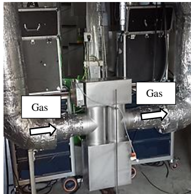
Fig. 2. ESP-L precipitator at the test facility, equipped with wood-chips boiler
