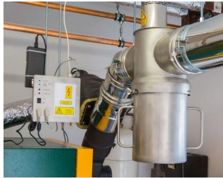
Fig. 10. Compact electrostatic precipitator downstream a wood combustion boiler
