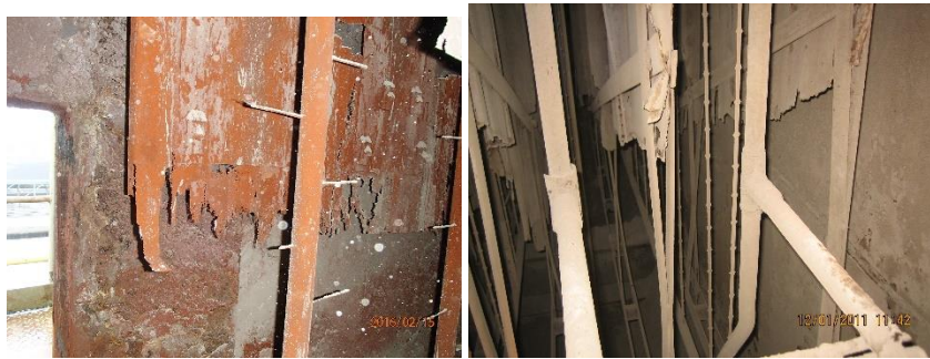
Fig 2. Corroded electrodes in second fields of ESP's with skewed flow model and frequent low boiler loads.
