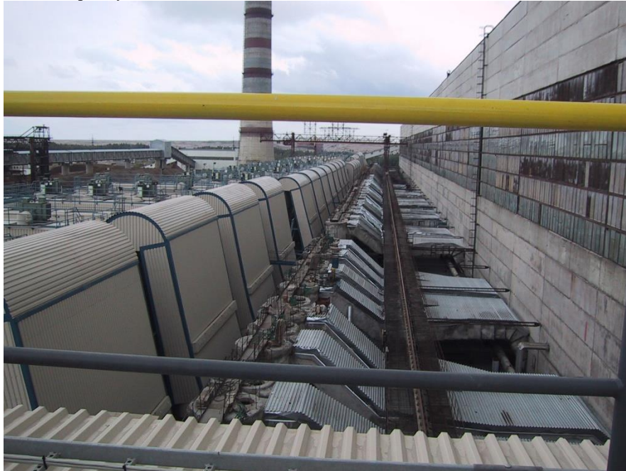
Fig 5. Example of inclined inlet flue gas ducts before the ESPs.
