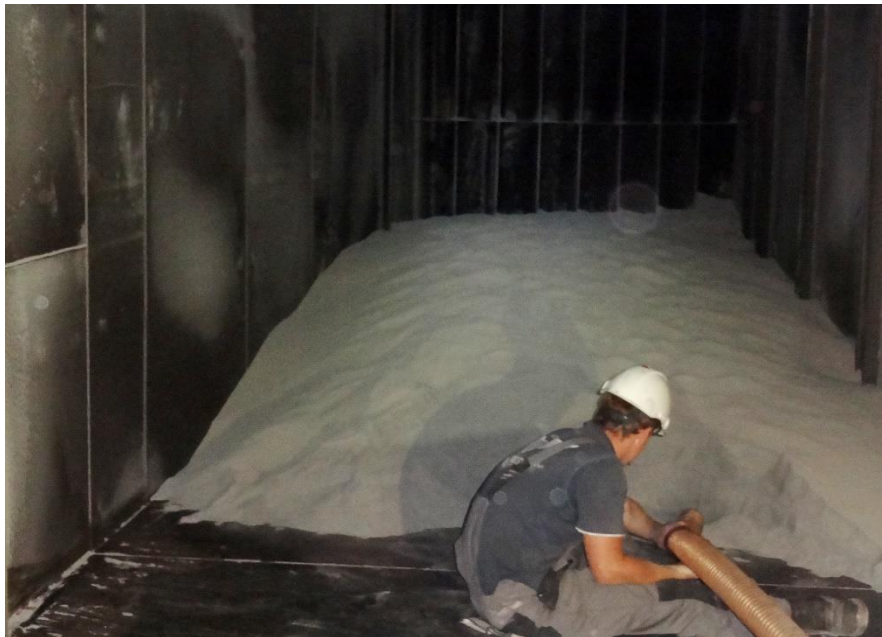
Fig 4. Manual evacuation of large dust deposits from horizontal gas duct shown in Fig. 3.
