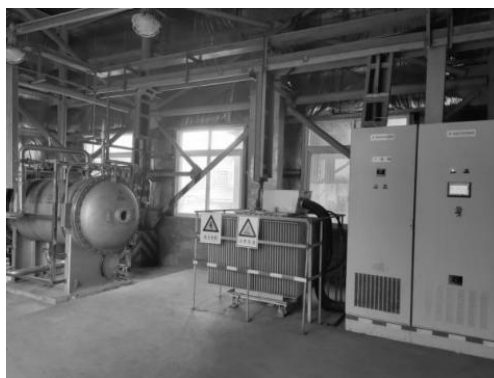
Fig.10. Variable frequency power supply applied to ozone generator
